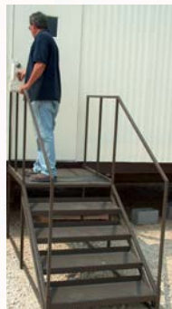
Prefab metal steps with landing and handrails.
